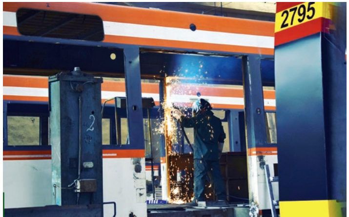
Employees of MPK Łódź Engineering Plant have knowledge and skills enabling them to carry out current repairs and general overhauls of the tram rolling stock
